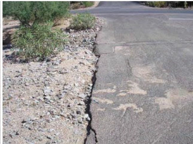
Edge Erosion from Stormwater Runoff
