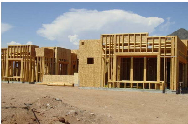
Wood frame residence under construction. Upon completion of construction, disturbed area around home will be revegetated with low water use plant material.
