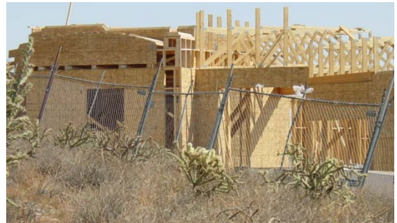
During construction a temporary chain link fence shall be installed to protect native desert from being damaged
